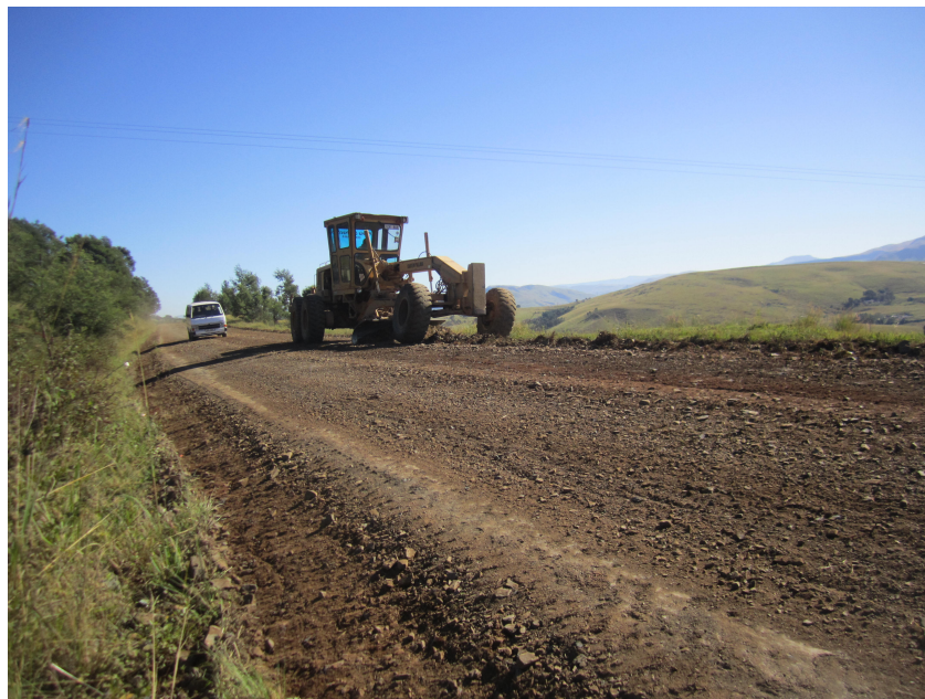
Plate 7: One of the main roads to Sandanezwe being cleared for further construction
